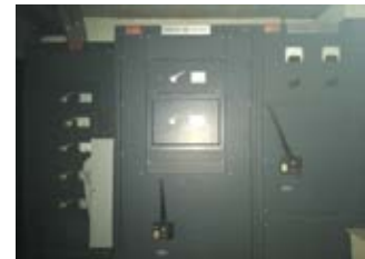
Auditorium Electric Service
