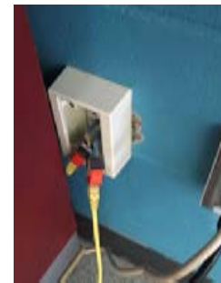
Loose Data Jacks
