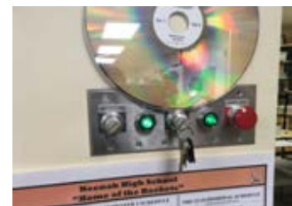
Science Room Power & Gas Shut-off
