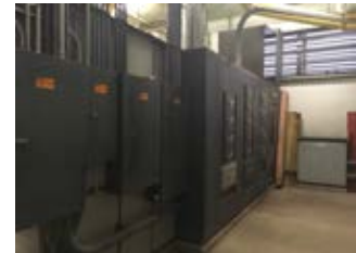
South Electric Service
