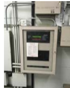
Fire Alarm Control Panel
